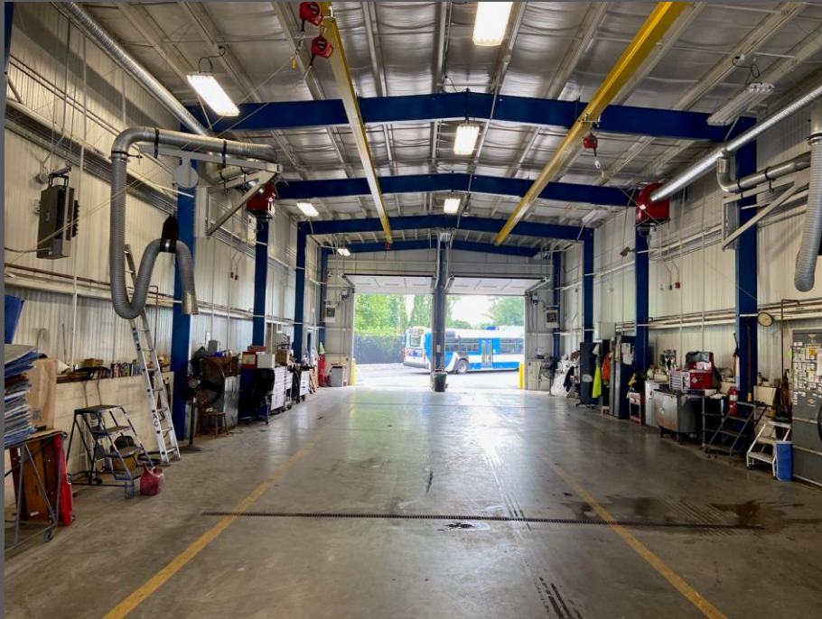
Building charging infrastructure at CTtransit Hartford facility
